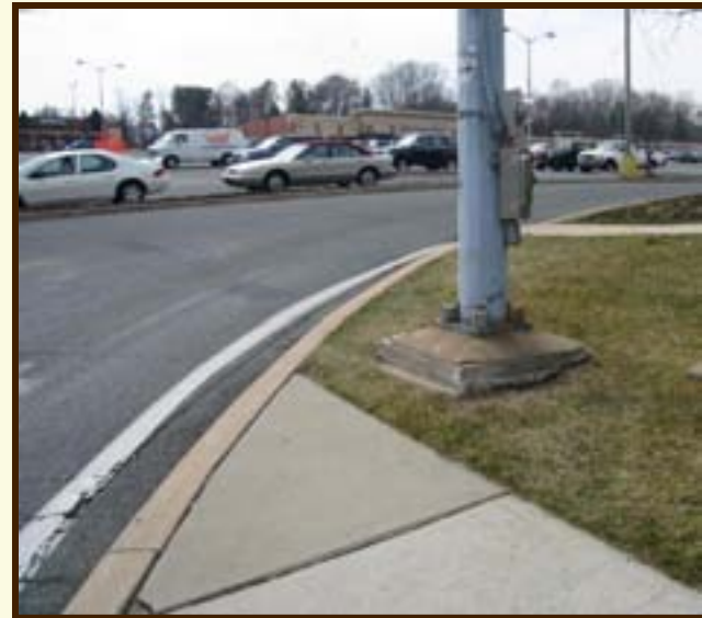
Several Intersections Lack Pedestrian Ramps
