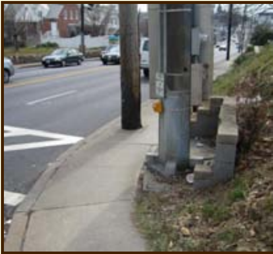
Many Utility Poles are Currently Placed in the Middle of the Sidewalk
