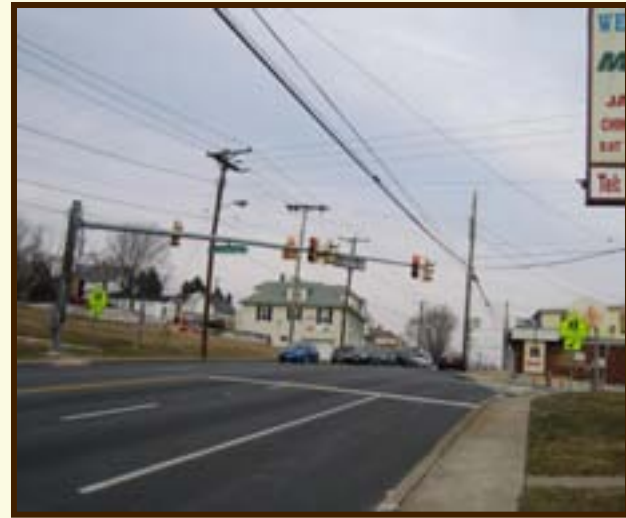
Typical Overhead Utility Configuration
